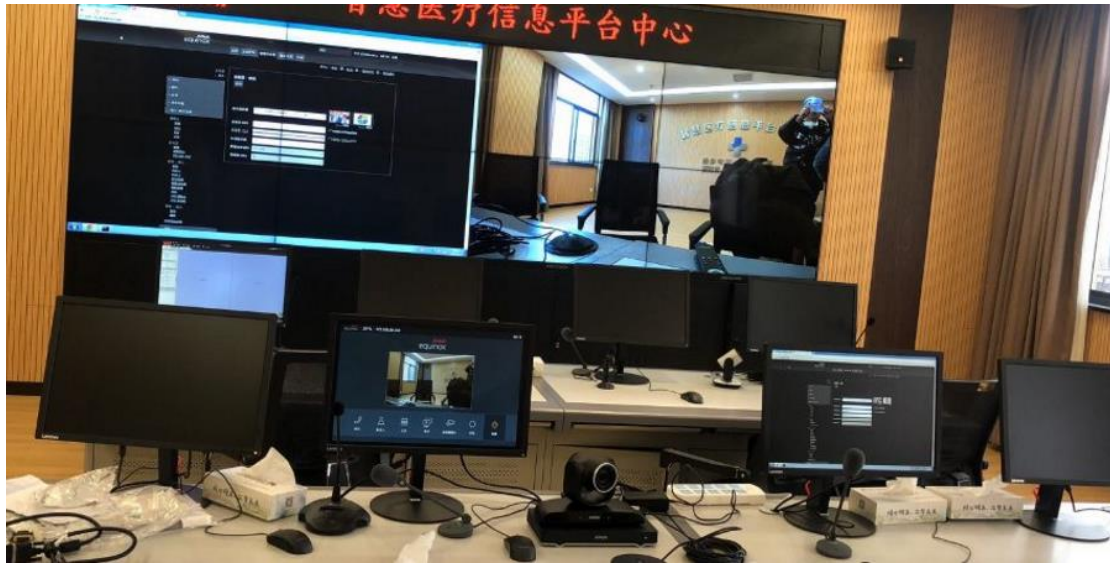
The equipment donated by Avaya deployed in the hospital's information platform centre
